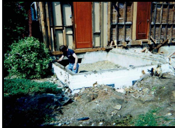
Side of building showing the original construction and an add on from a later date.
