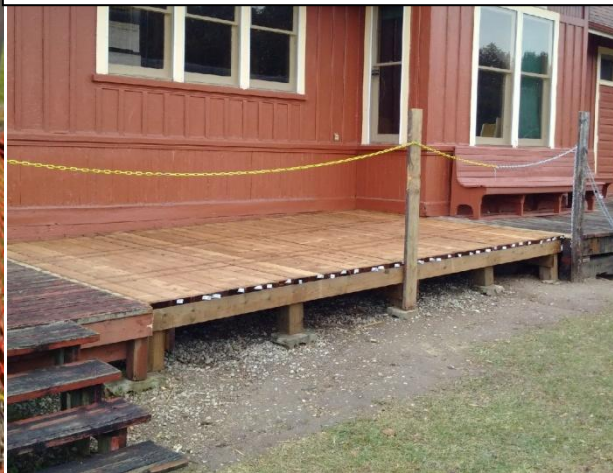
Deck section nearly completed. The ramp is gone and been replaced by a gradual slope. Looks great!!
